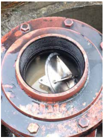
Investigation to see if the new 6-inch sewage air/vacuum valve was destroyed.
