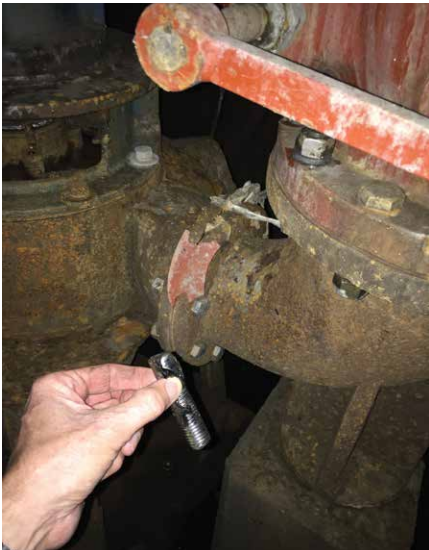
Pump discharge flange damaged and bolts sheared off between discharge 90 and check valve.
