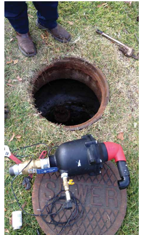
The field evaluation of the sewage force main determined it was necessary to install a transient monitoring system on the air/vacuum release valve.
