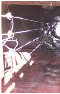
Optifloats installed in wet well.
